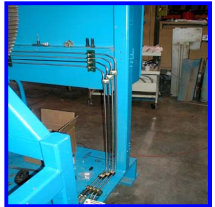
Views of tubing conversion
